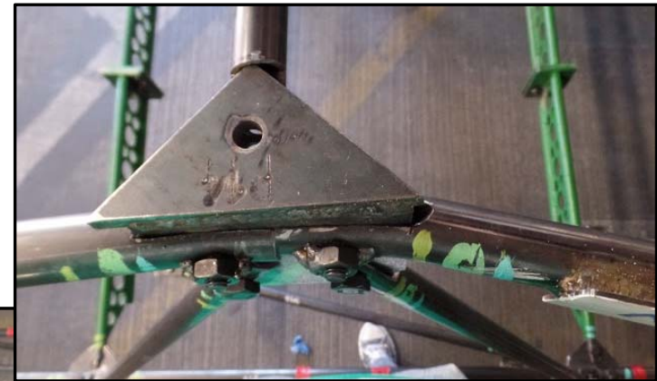
Figure 19: Right connection pipe failure [3]
